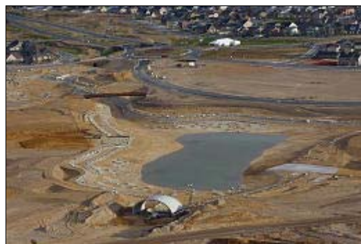
Water is pouring into the first phase of Oquirrh Lake at the Daybreak project. The lake will take an estimated five years to finish.
