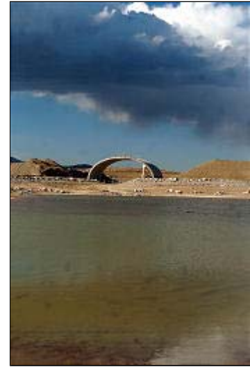
One of the project's two vehicular bridges is being built with a 26-foot clearance to allow for boats.
