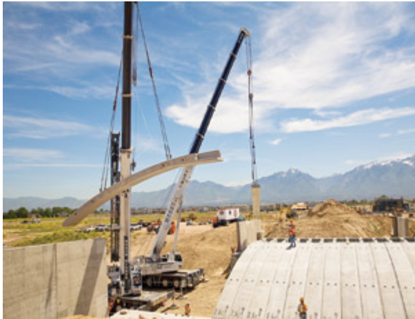
Photo Courtesy Of Kennecott Land Precast arches made out of recycled concrete were built on site, not shipped.
