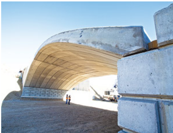
Photo Courtesy Of Kennecott Land Builders of a Utah community bridge want a green rating.
