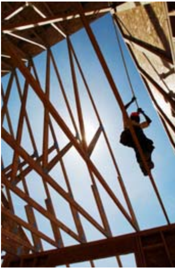
Antonio Torres frames a house in the 4,200-acre project in the southwest Salt Lake Valley. It will eventually have 13,000 homes.
