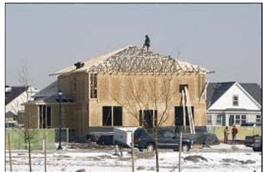
Construction crew works on a home in the Daybreak development. Housing starts rose 17% in the fourth quarter.
